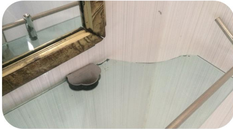
Badly Maintained Premises
